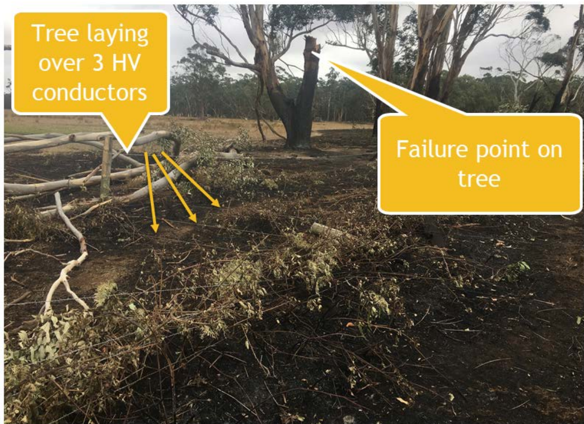
Figure 3: Tree failure showing HV conductors on the ground
