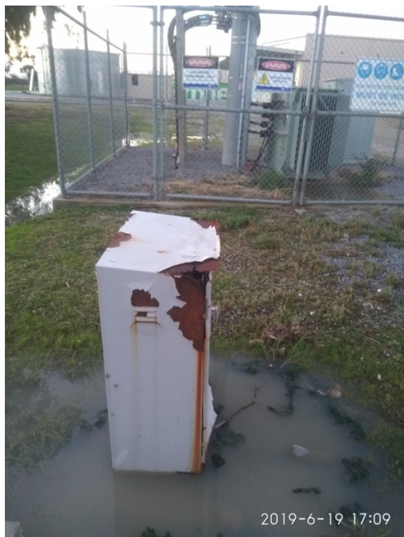
Figure 7: Example of equipment that is poorly maintained and in an unsuitable location
