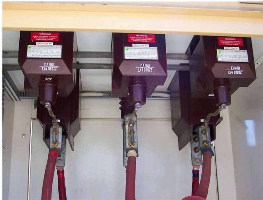
Embedded metering transformers
