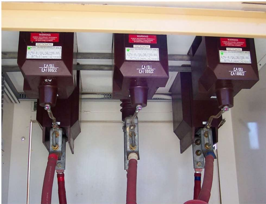
Embedded metering transformers
