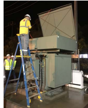
GFN - Arc Suppression Coil
