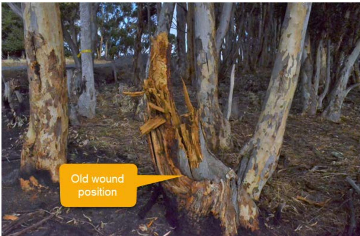
Figure 4 shows that the failure point of the tree limb is located above an old wound where the tree had been cut back prior, and subsequently regrown. The ESV arborist on site noted this as a point of structural weakness in the tree.
