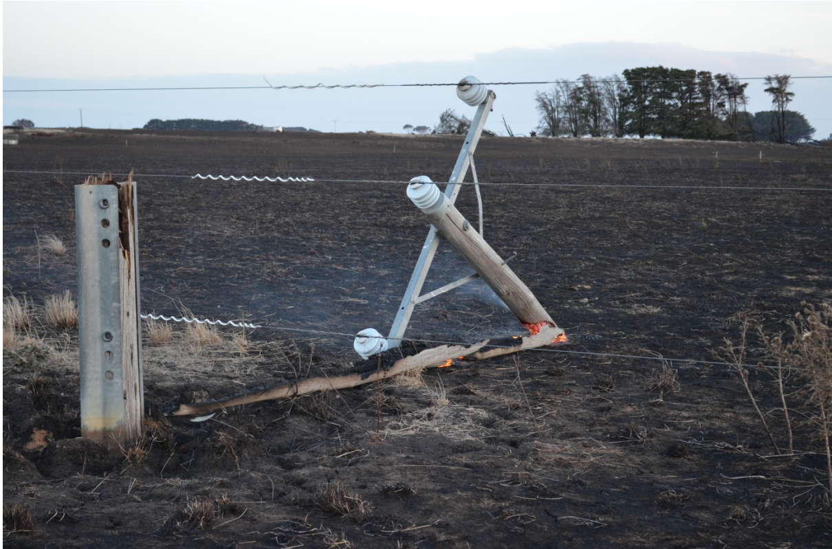
Figure 7: failed Pole 4, 974 Sisters-Garvoc Road
