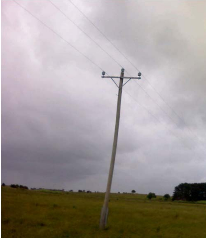
Figure 1: Pole 4 prior to failure (taken 5 December 2012)
