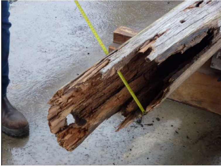
Figure 9: Pole 4 cavity and termite infestation
