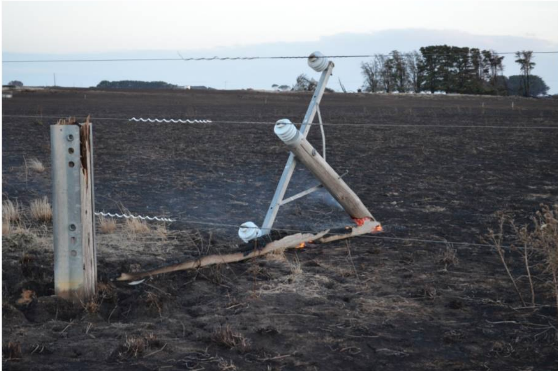
Figure 7: failed Pole 4, 974 Sisters-Garvoc Road
